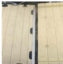
Gangway connection to dock
